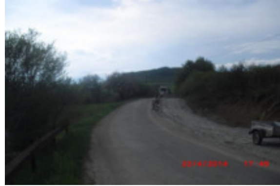
Photo.2. DJ 108 B, the section affected by slip
